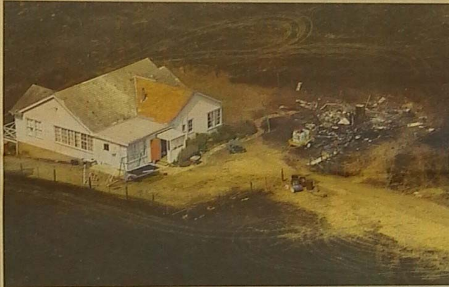
BLACK DAY: The shed is destroyed and the paddocks are a charred mess... but mercifully this house near Edenside survived this week's fires. Picture: TONY PALMER
